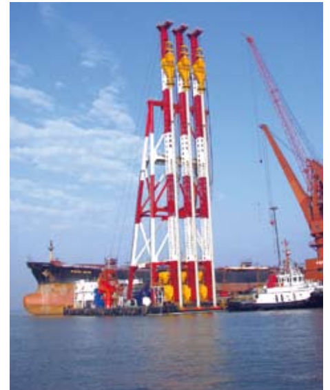
■ 港珠澳大桥挤密砂桩项目 Hongkong-Zhuhai-Macao Bridge (Sand Compaction Pile Construction project)
